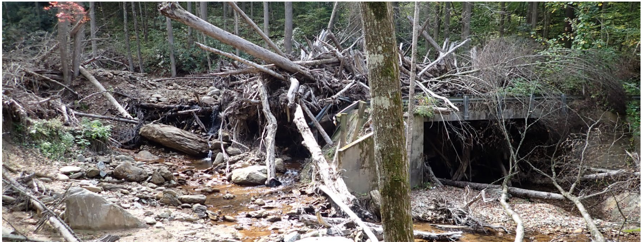
Figure 1: Bridge failure due to wood debris and alluvium accumulation in the Dillingham Creek watershed.
