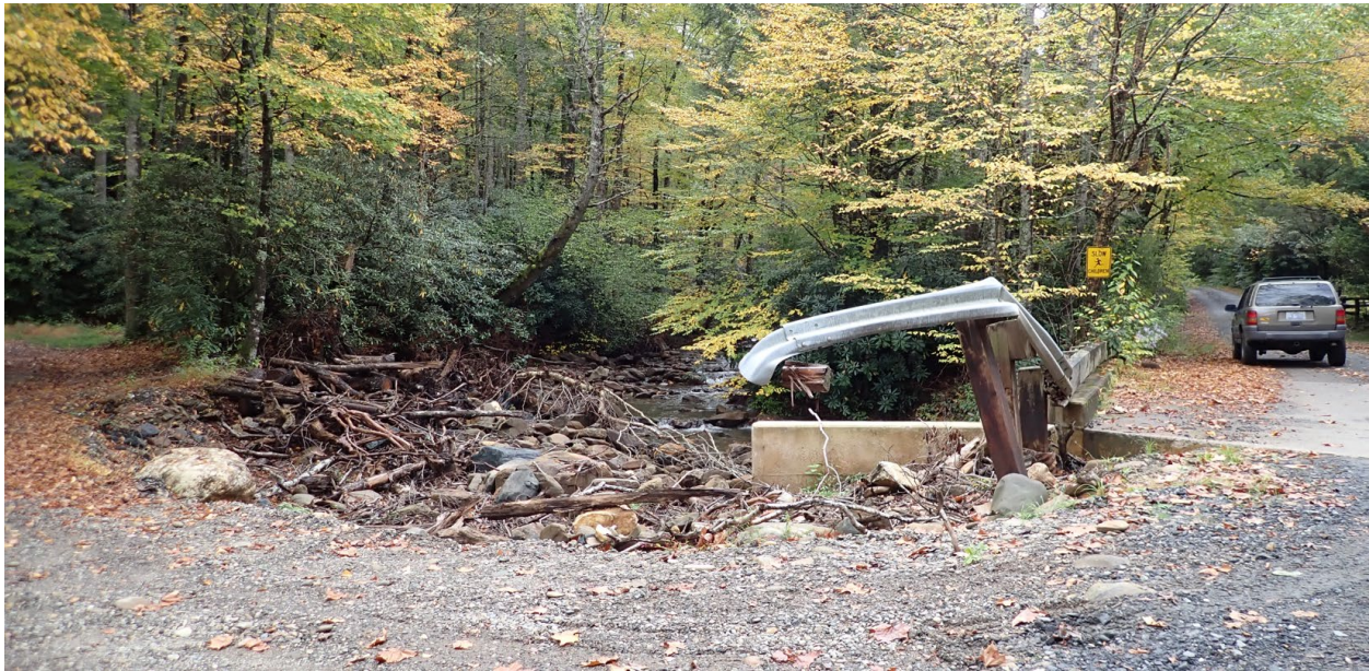
Figure 21: South Toe River Road (NFS-472) crossing of Big Lost Cove Creek (site ID: BLC-1), in the South Toe River watershed. Design flood discharge ( Q_{dfd} ) = 1360 cfs (flood potential method: Q_{efp} ). Q_{100\text{ Index}} = 2280 cfs; Q_{100\text{ regional regressions}} = 751 cfs.
