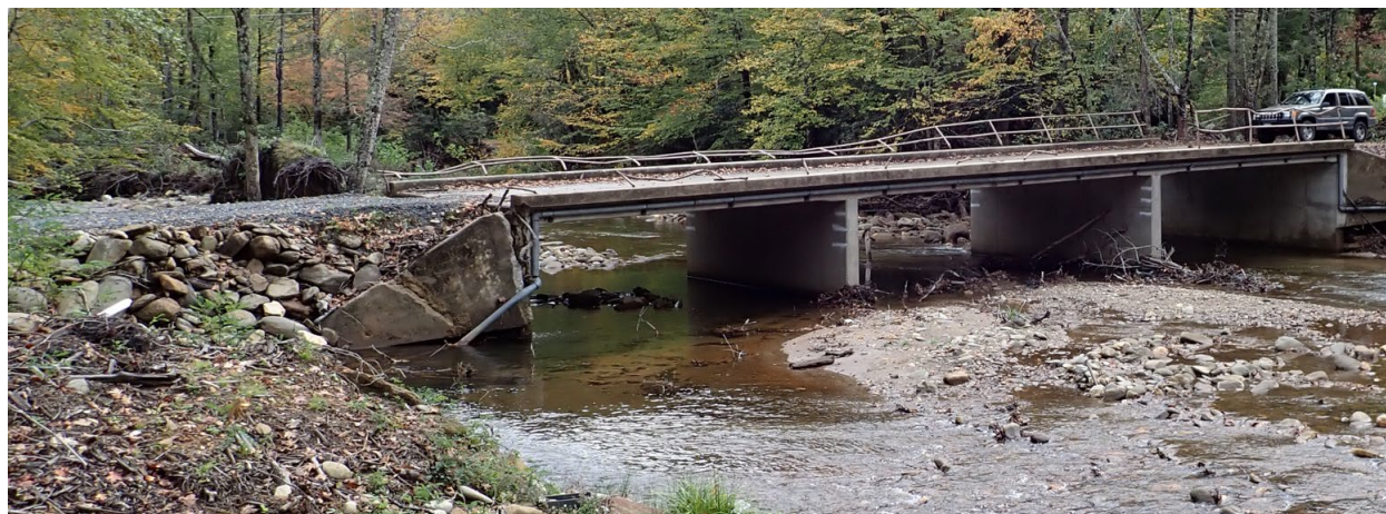
Figure 8: Heavily-damaged bridge over the South Toe River, at the Black Mountain Campground on the Pisgah National Forest.
