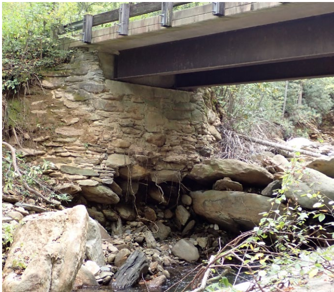
Bridge abutment scour in the Curtis Creek watershed
