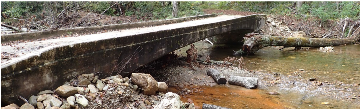
Figure 2: Damaged bridge over the South Toe River.
