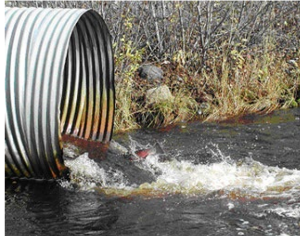
Figure 49: Culvert outlet drop, with Coho.
